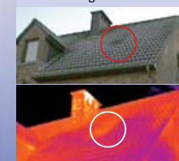
The infrared inspection locates missing insulation in the roof. This can now be repaired and further energy loss prevented.
